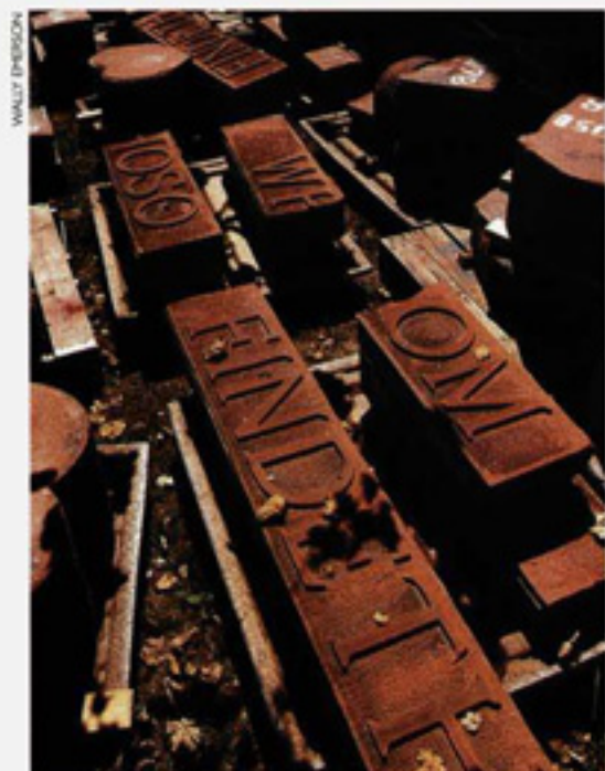
FINDETH WISDOM: Stones from the front of Spooner Hall have been removed and refurbished as part of a renovation of the old campus building (see Hiltopics sidebar, p. 11). When reassembled above the triple-arched entryway, these stones will read, "Whoso Findeth Wisdom Findeth Life."
