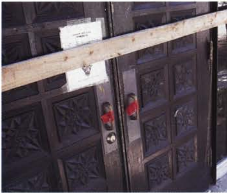
NOBODY'S HOME: High weeds (p. 32) and boarded doors on Stewart Avenue.
